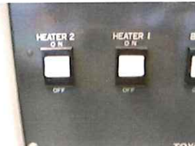
HEATER 1 ON, HEATER 2 ON
